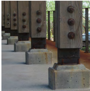
Wooden posts + steel hardware
