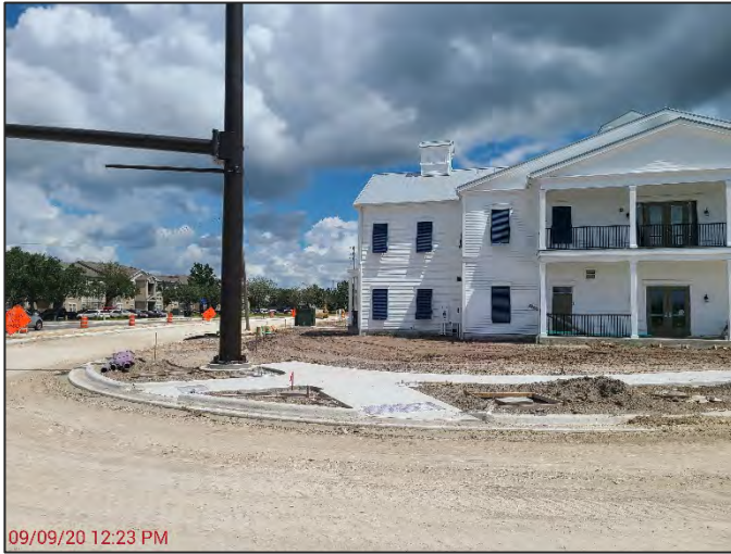
Photograph 1. View of Partin Settlement Road and Shady Lane intersection on east side of APE, looking north.
